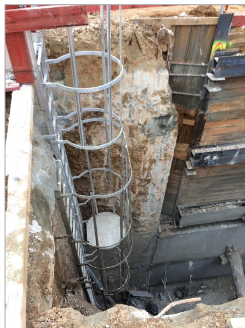
Safety cage ladder equipped with retractable bearing.
